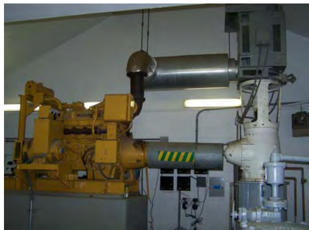
Example – Auxiliary Engine at well site for back up power source in the event City power is temporarily unavailable
