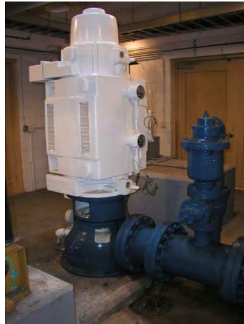
Example - Well Pump and Motor
