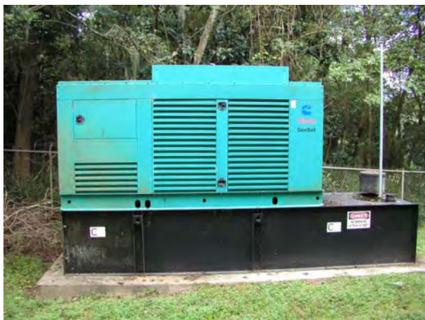
Example – Generator at well site used for back up power source in the event City power is temporarily unavailable
