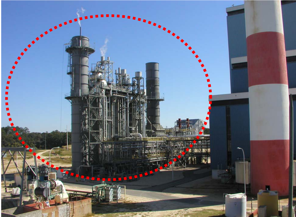
This picture shows the majority of the constructed equipment added to repower Hopkins Unit 2.
